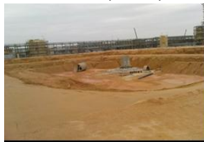
C3 – Flue-Gas Desulphurization (FGD)
