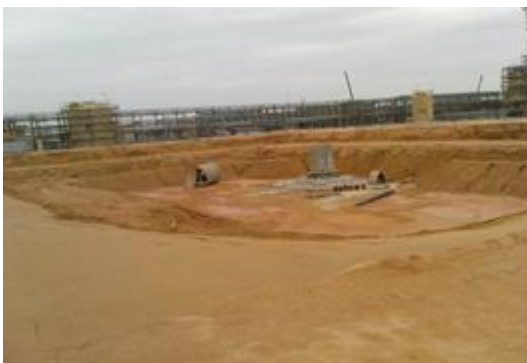
C3 – Flue-Gas Desulphurization (FGD)
