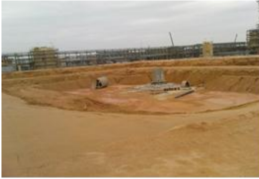
C3 – Flue-Gas Desulphurization (FGD)
